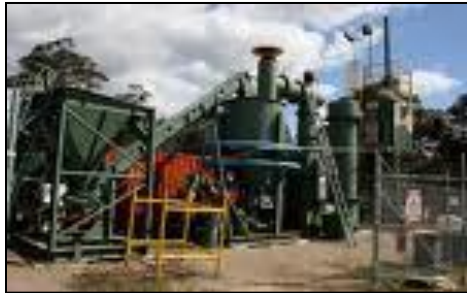
3 MSW plant 1,200tpd capacity
